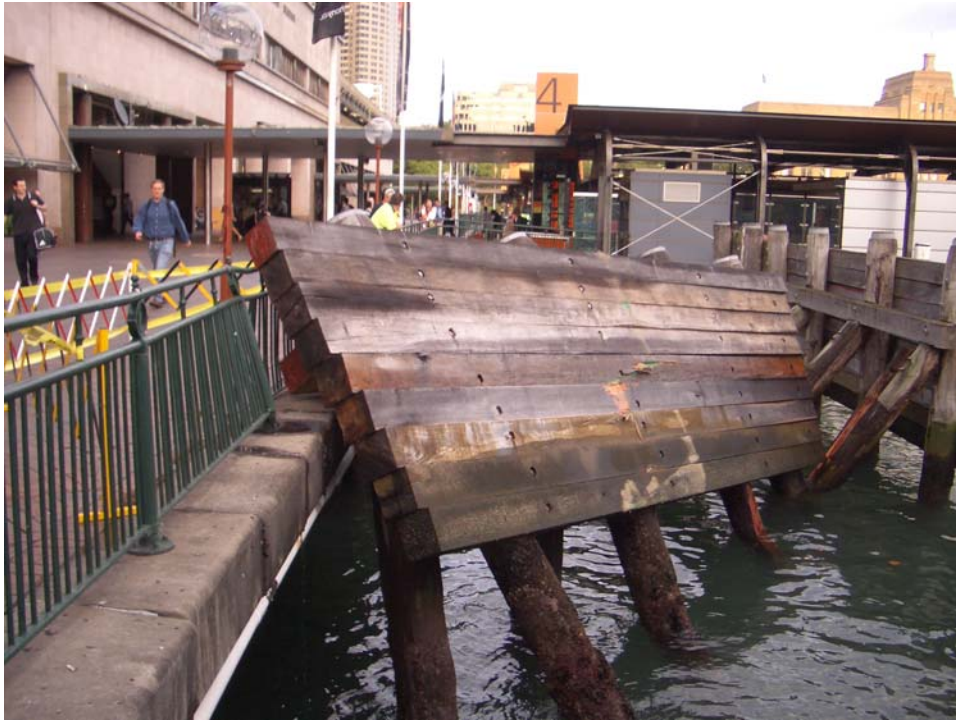
Figure 2: Damage to the Backboard at No. 3 West Wharf
