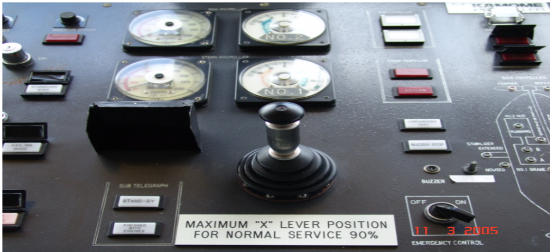
Figure 7: Showing the X-Y lever and Emergency Control Switch
