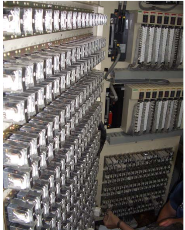
Figure 10: Part of the Kamome propulsion control circuitry
