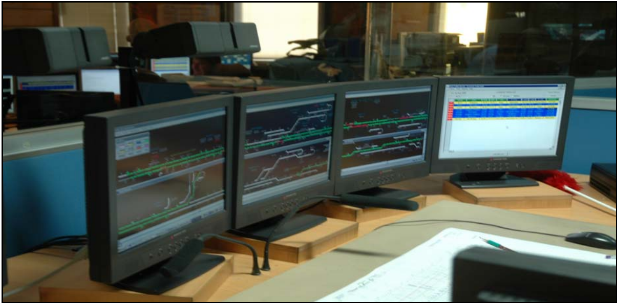
Photograph 6: Train Controller's Indication Panel at HTCC. (Photo supplied by ARTC)
