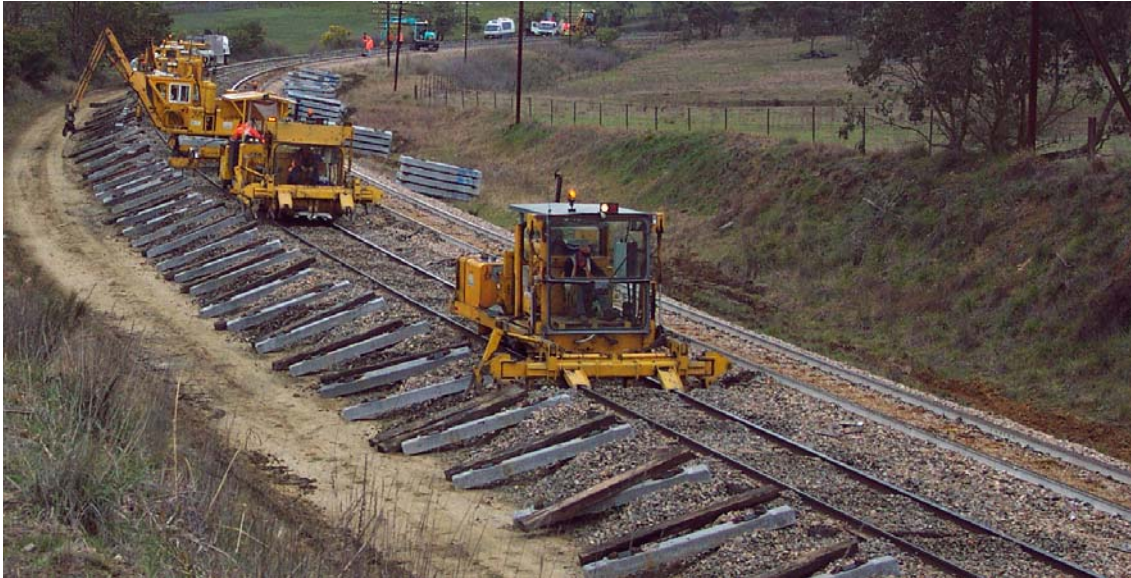
Figure 3 – Installation of low profile concrete sleepers in a production line (scarifier machines in foreground)
