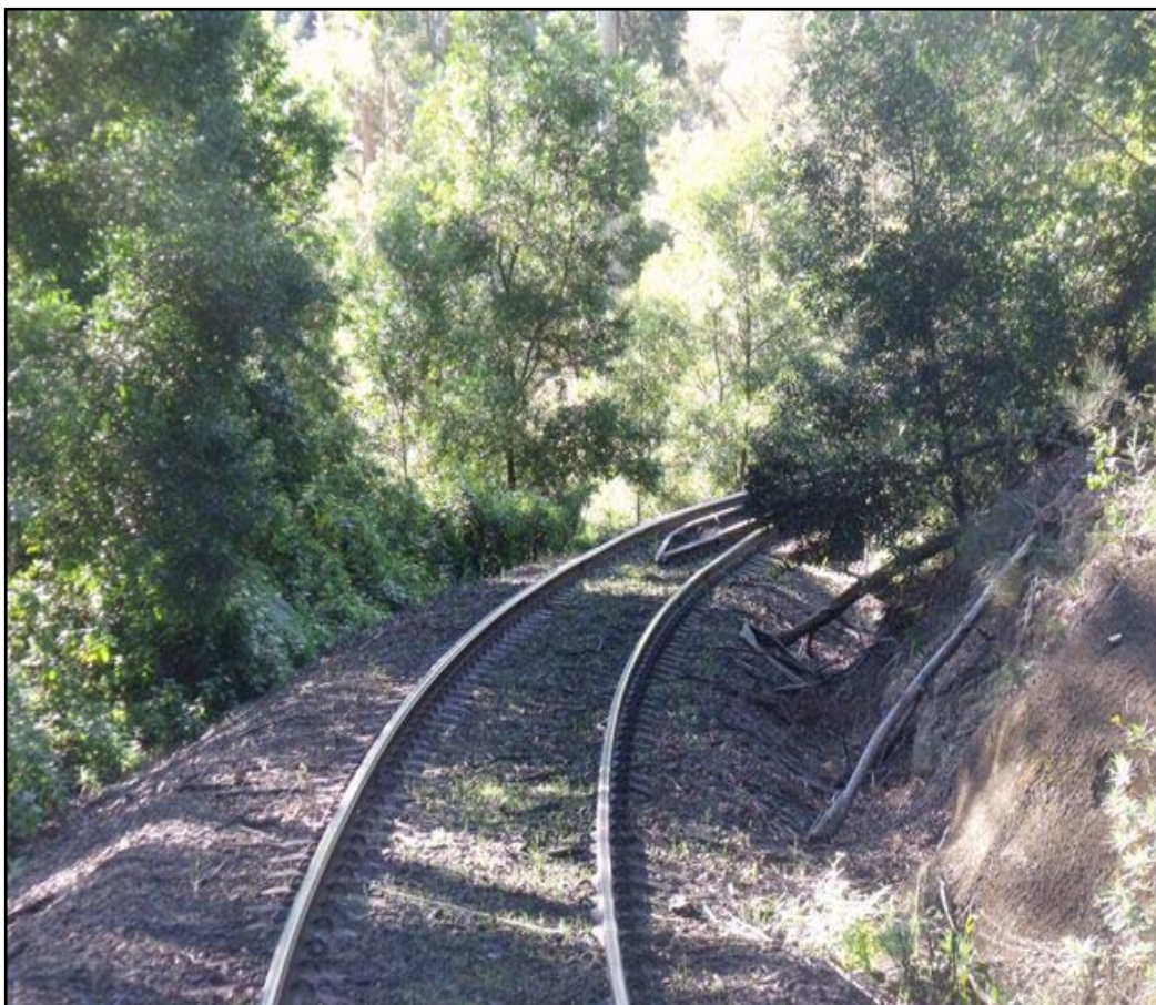
Photograph 1: View along the last curve on the approach to the viaduct (Country end)
