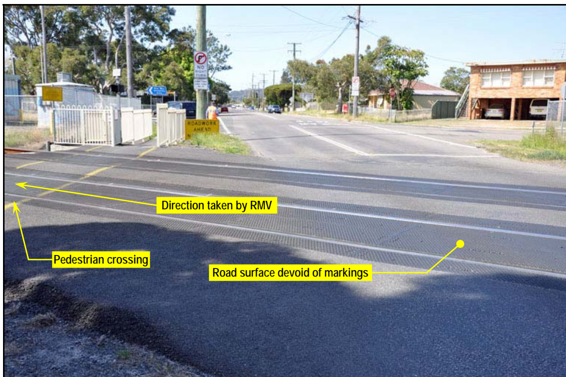
Photograph 10: Crossing surface devoid of road markings
