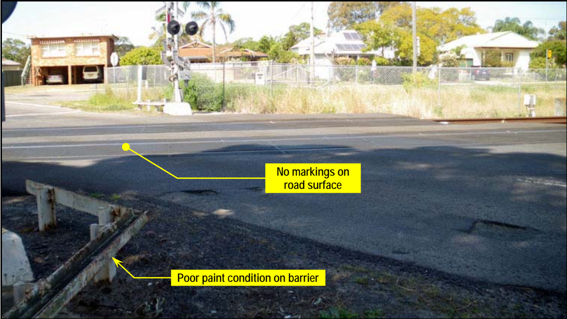
Photograph 11: Condition of barrier paintwork and road surface inside rail corridor
