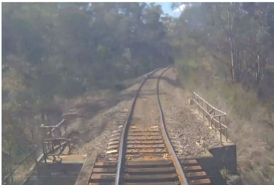
Figure 2: View of the track buckle (367.538 km) at Bylong Valley Way overpass
